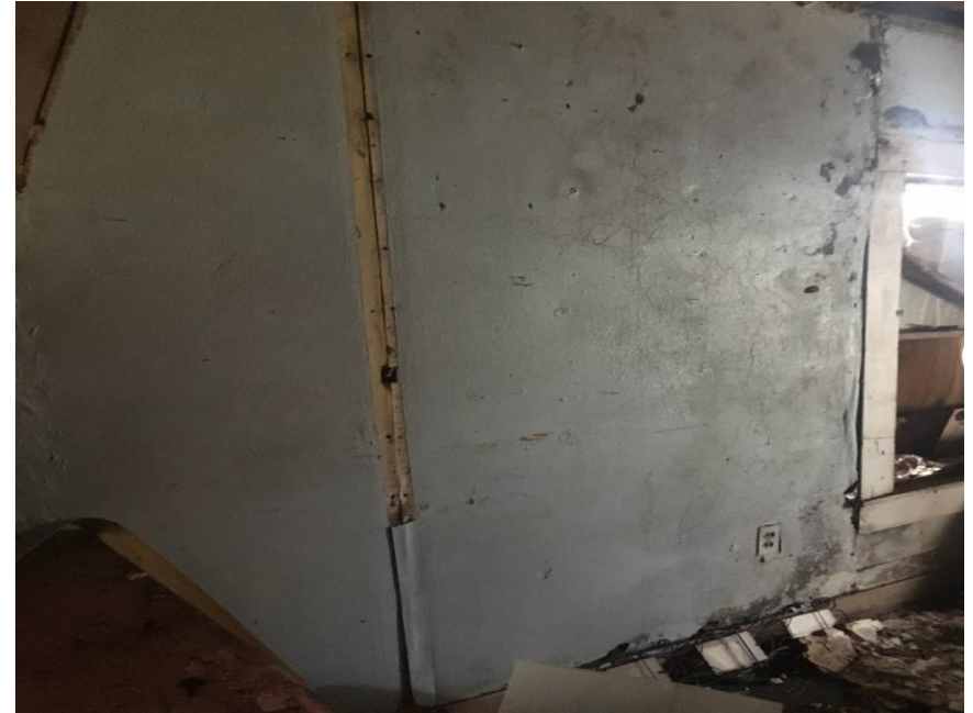
Photograph No. 2 View of HA-02: White Sheetrock, Tape & Mud-Wall
