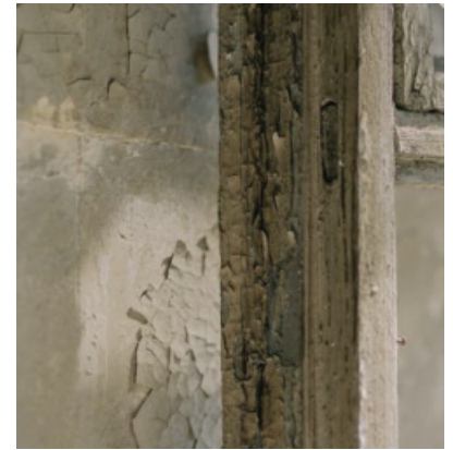
If there is flaky paint like this in your house, don't touch it! It may contain lead hazards!
