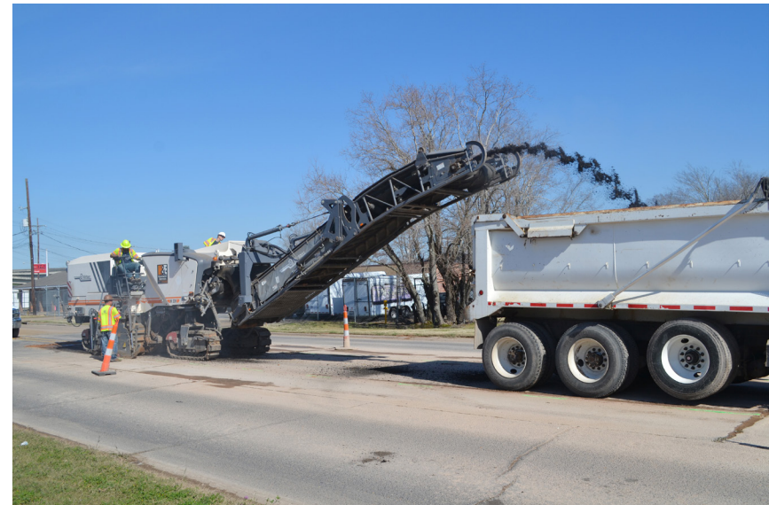
Workers with Gilchrist Construction continue working to remove old roadway on Upper Third Street between Monroe Street and MacArthur Drive.
