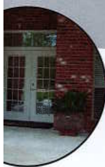
Minimum clear door width required, as well as beveled threshold and usable hardware.
