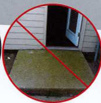
The step at this entrance landing makes this building inaccessible.
