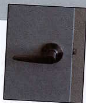
This exterior door hardware is compliant as it does not require pinching or twisting.
