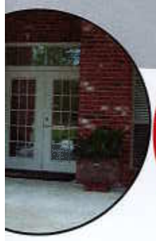
Minimum clear door is required, as well as a beveled threshold and usable hardware.
