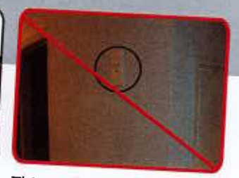
This outlet is non-compliant; it is placed above 48".
