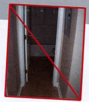
This 22" doorway is non-compliant; Doorway must be at least 32".
