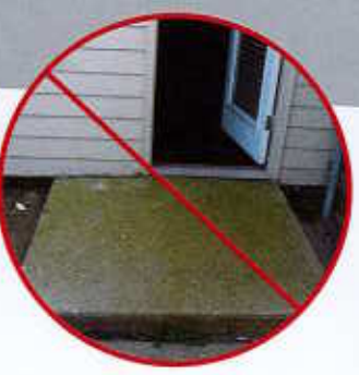
The step at this entrance landing makes this building inaccessible.
