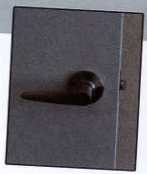
This exterior door hardware is compliant as it does not require pinching or twisting.
